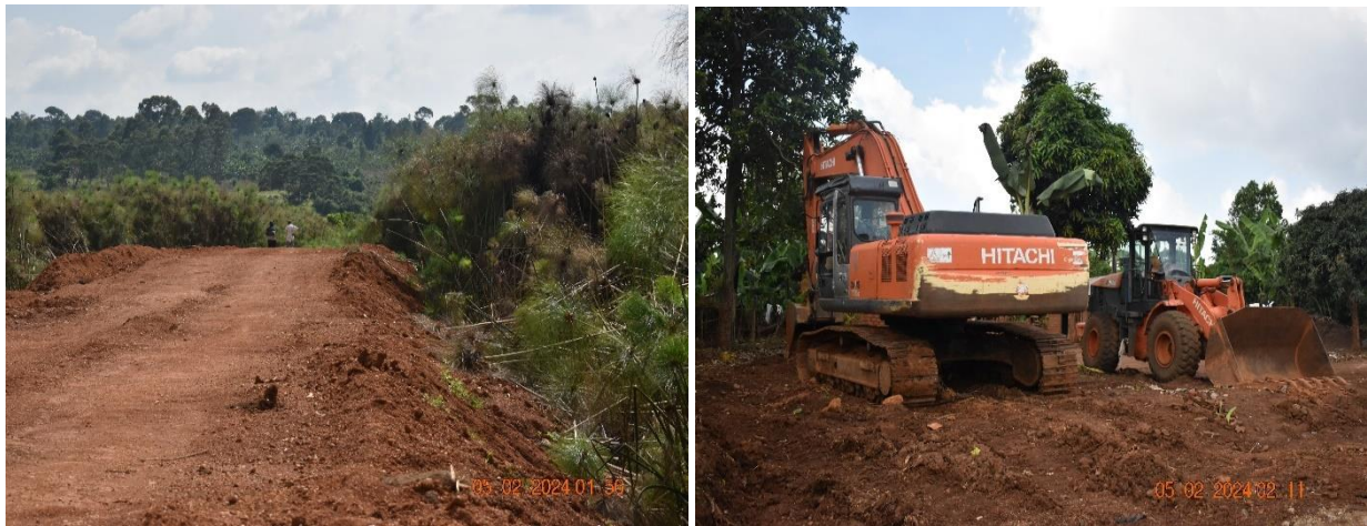
Halted works at 50% progress for agricultural access road (left) and broken equipment (excavator and tractor) for operation awaiting overhauling at Kitanga Village, Kimanya Sub-county
