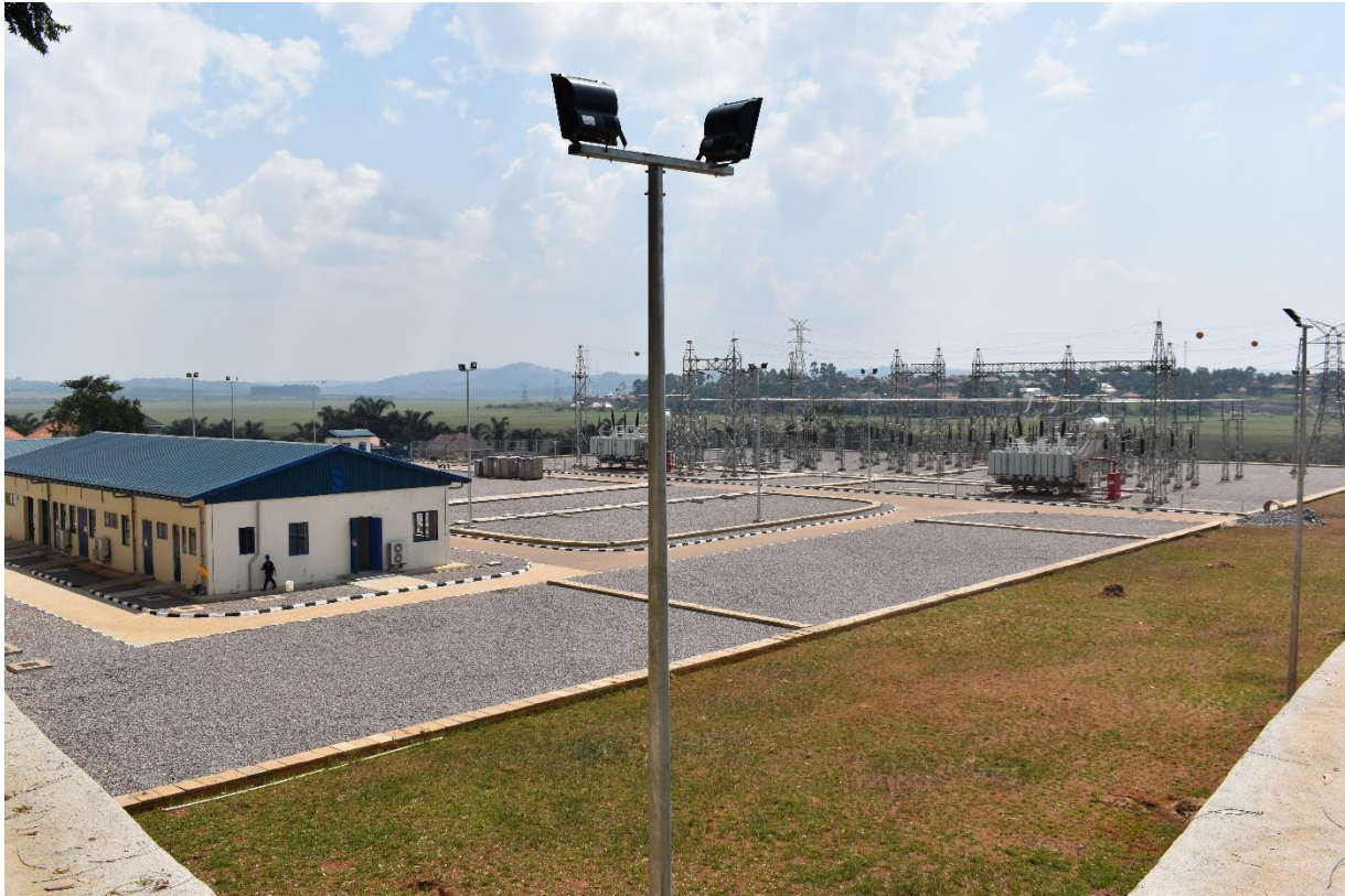
Completed 132/33kV Entebbe Substation
