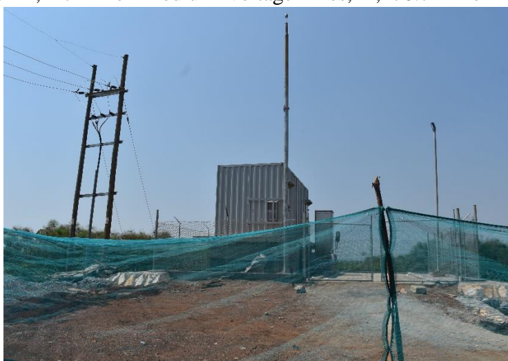
One of the two installed switching station for Bugala marine cable at Bukakata
