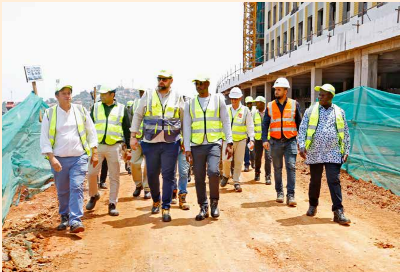
PSST Ggoobi, his Deputy Ocaillap and other technical team visiting Lubowa hospital to assess progress of construction works
