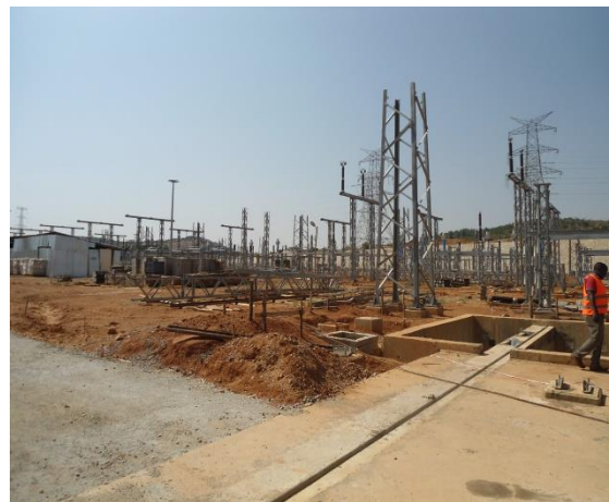
Abandoned project site at Mirama Hills
