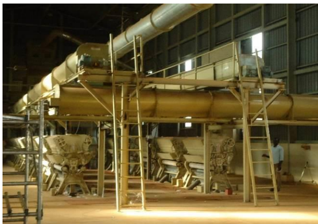
Installed and functioning machinery that required new delinter and grading machines at Pajule Ginning Factory in Pader District for increased production
