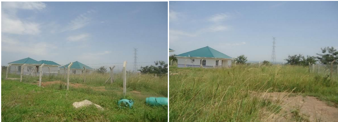
Unmaintained, completed Animal Disease Control Centre in Got Apwoyo Sub-county, Nwoya District
