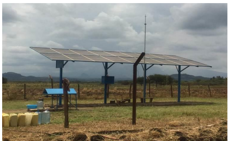
NAADS solar powered irrigation system was installed in Kween District and was functional
