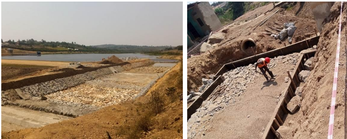
L-R: Overview of the dam and spillway; Culvert works ongoing at the access road destroyed by the floods at Kyenshama dam
