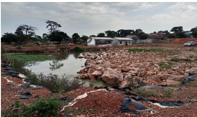
Stalled works at Kiyindi landing site in Buikwe District
