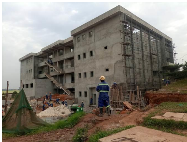
MAAIF financed National Metrology Laboratory was under construction at the UNBS Headquarters in Wakiso District
