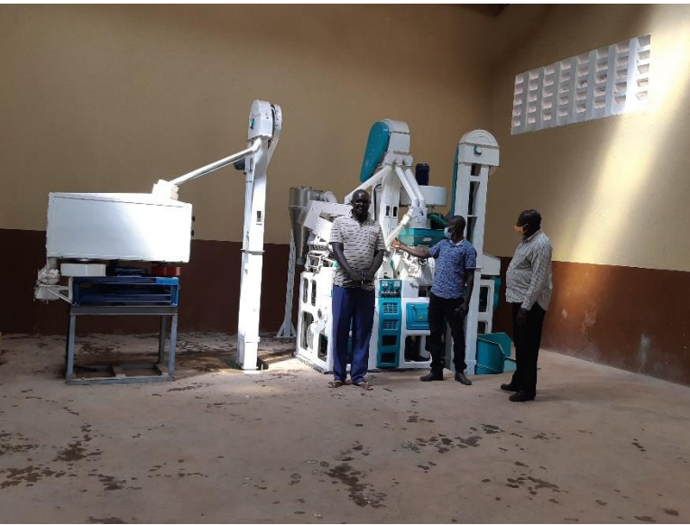
Installed rice huller at Amuru Tek Livestock Cooperative Miller
