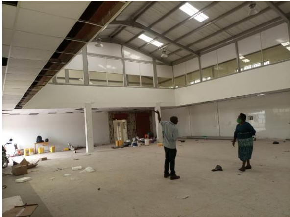
Works for the milking parlour at NALIRRI in Wakiso District near completion
