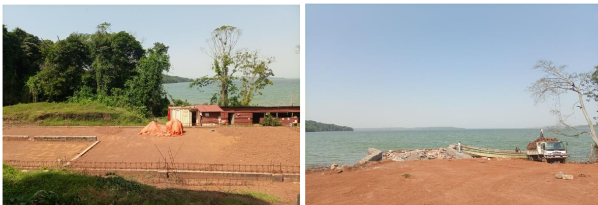
Works at Bugala ferry landing site in Nkusi Village by MAAIF had stalled for more than three years (left) and ongoing construction works by UNRA whereby 90% of loading jetty was complete
