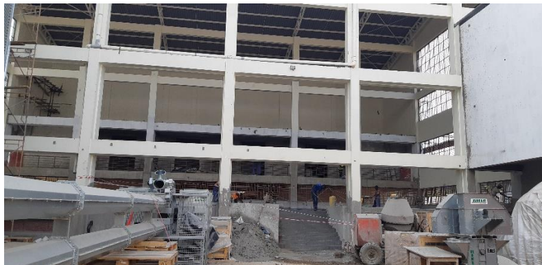
Top-Bottom: Silos installed and construction works ongoing at Soroti High Value Addition Facility
