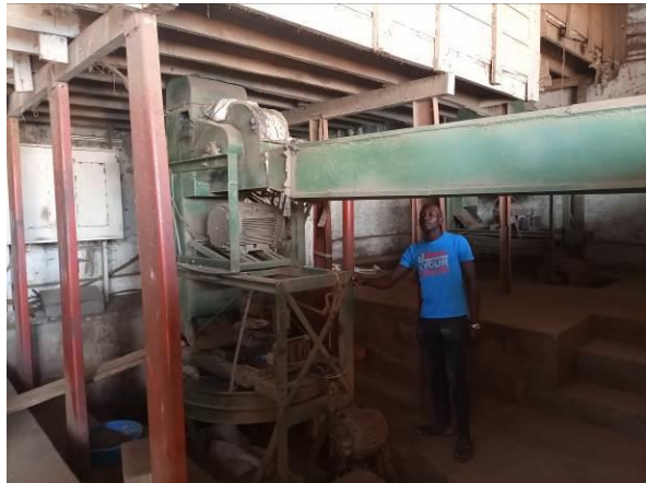
ACF financed machine installed in coffee factory in Kizigo village Masaka district
