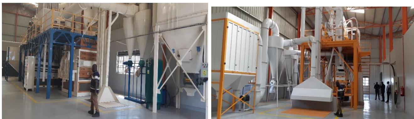
L-R: Equipment for maize milling among others and packaging and equipment for millet, sorghum among others processing and packaging in Arua processing facility
