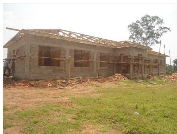
The hostel, planned to be completed in FY 2020/21 was still at roofing stage at Rubona Stock Farm in Bunyangabo District
