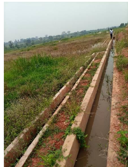
Completed civil works of irrigational system at NACRRI in Wakiso District; facility was not yet operational
