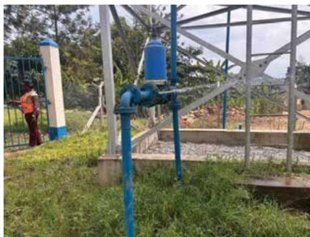
Leakages at the reservoir at Mpegwe Small-Scale Irrigation (SSI) Scheme in Mpegwe Village, Kikandwa Parish, Kakiri Sub-county, Wakiso District
