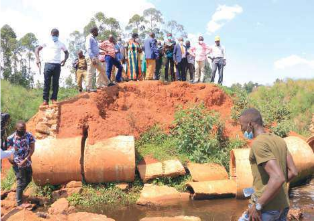
Hon. Peter Ogwang-Minister of State, Office of the President (Economic Monitoring) monitoring the Construction of a Bridge in Kagadi District in December 2021.
