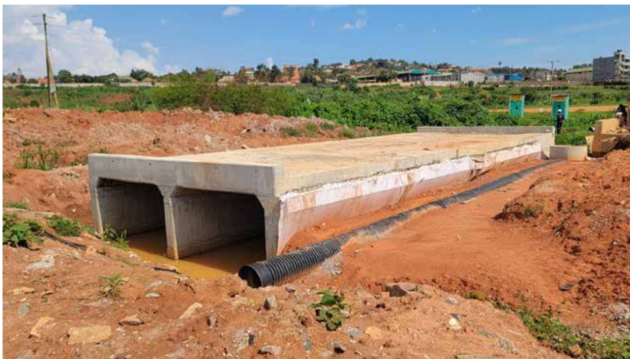
Top Left: Installed guard rails in the North Estate. Top right: Weigh bridge under construction in South A Estate. Bottom: A box culvert and sewerage line under construction in South B Estate in Kampala Industrial Park-Namanve
