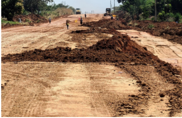
Koboko-Yumbe-Moyo: Road bed preparation activities of spreading and compaction of G7 material at Km 53+051 in Yumbe district
