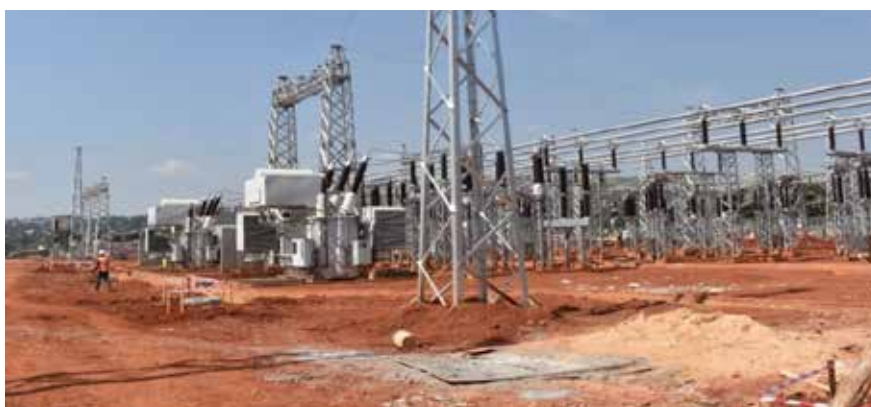
Installed equipment in the Buloba Substation switchyard at Nakirebe,
