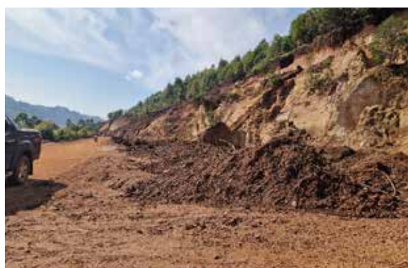
L: A section of Kabale-Lake Bunyonyi (15.1 km) road after clearing and grubbing at km 1+860
