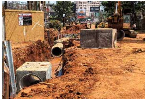
Ongoing drainage works at the Kabalagala Junction under Lot 1 in Makindye Division
