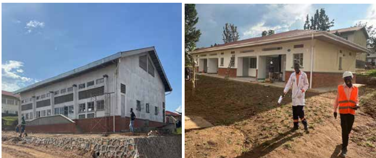
Left to right: Ongoing completion works for the multipurpose hall and the four-unit staff house at Lwengo Technical Institute in Lwengo District.
