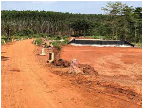
A constructed box culvert at Km 6+225A along the Mpigi-Muduma road in Mpigi District
