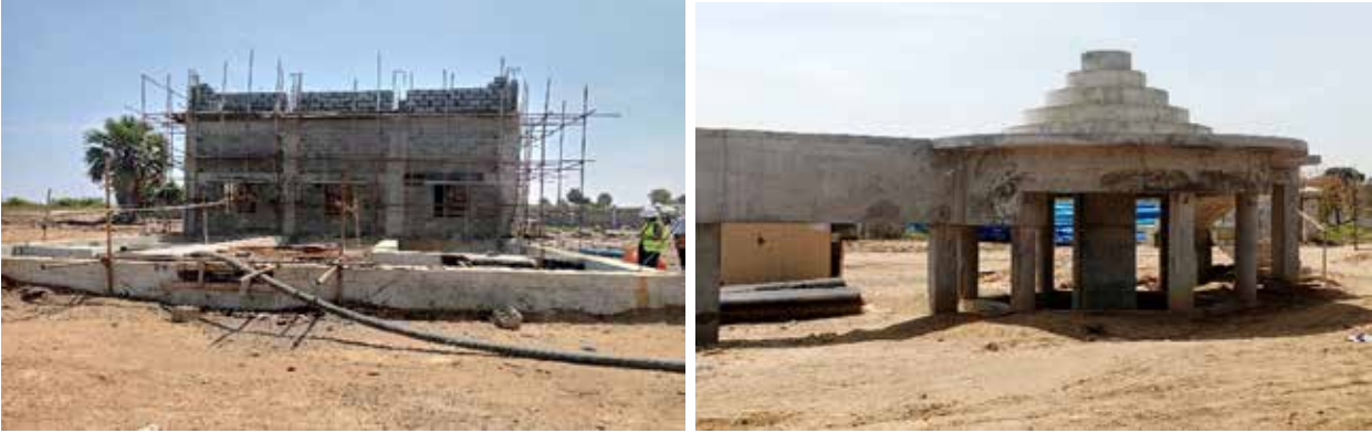
L: A raw water sump and pump house; R: Aeration structure for Adjumani WSS in Adjumani District.
