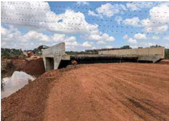
A completed bridge with ongoing road works on the approach roads in Wakiso district at Km 5+200 along the Sentema 2 road of Lot 5
