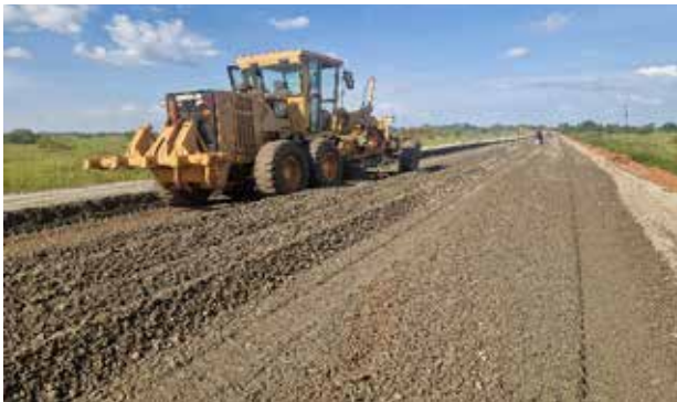
Construction of the base layer at Ibutje Swamp, km 72+150 Along Rwenkunya – Apac Road Project
