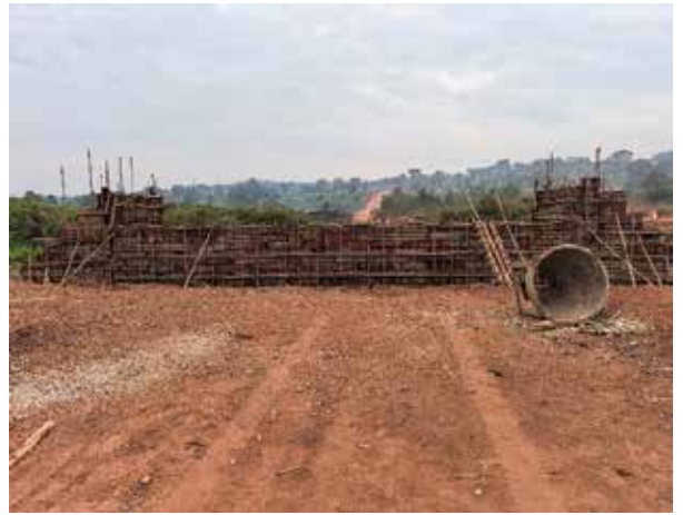
Ongoing construction works on box culvert at Km 5+187 along the Bukasa-Sentema-Kakiri road in Wakiso District
