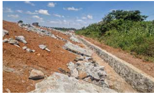
Stone pitching of the side slopes and side drains at km 180 + 240 along Apac-Puranga Road Project
