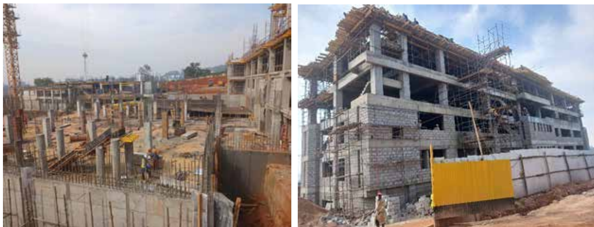
L-R: Ongoing work at Block A and B at Uganda Heart Institute
