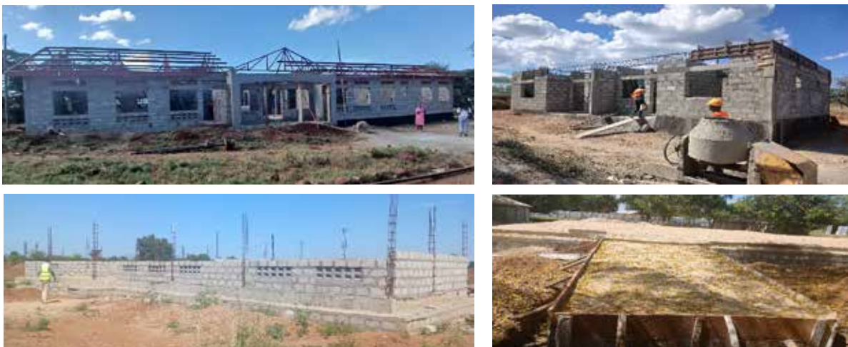
Clockwise: Maternity ward at Rupa HCII (Moroto) Staff house at Lorengdwat HCIII (Nakapiripiti) Operating theatre at Nabilatuk HCIV and Maternity ward at Akuyam HCIII (Nakapiripiti District)
