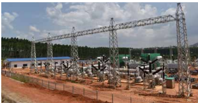
Installed switchgear, gantries and transformers at the Mukono
