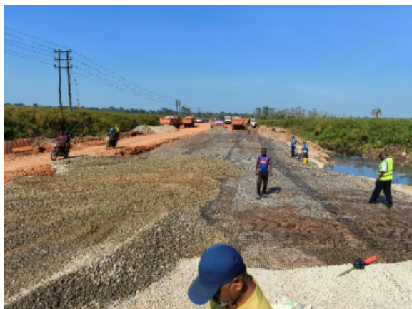
Luweero-Butalangu: Laid geogrid material in a swamp section of the Lugogo River between Km 7+900 to 8+400 at the border of Luweero and Nakaseke districts
