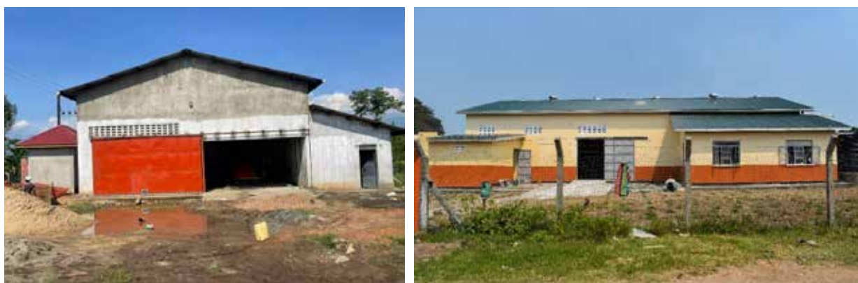
L-R: On going civil works at Gatyanga Coffee Processing plant in Bunyangabu District; R-ongoing construction of Ocorimongin rice processing factory in Katakwi District
