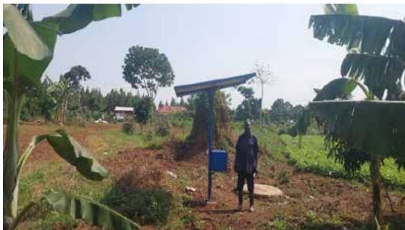
Pole-mounted solar system with submersible irrigation pump at a farm in Buwama, Mpiigi district.
