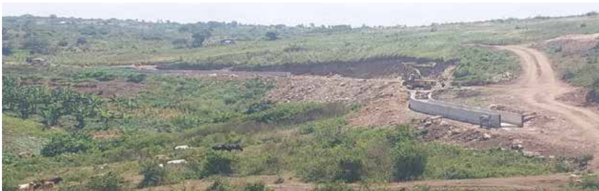
On-going civil works on the open water channel for the Hoimo mini-hydro project
