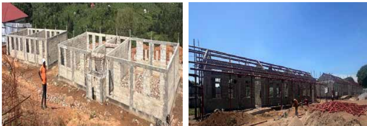
Left-Right: Ongoing construction of a science laboratory and classroom blocks at Nkondo Seed Secondary School, Nkondo Subcounty, Ibanda District, and classroom blocks at Budiidi Seed Secondary School, Budiidi Subcounty, Namayingo District.
