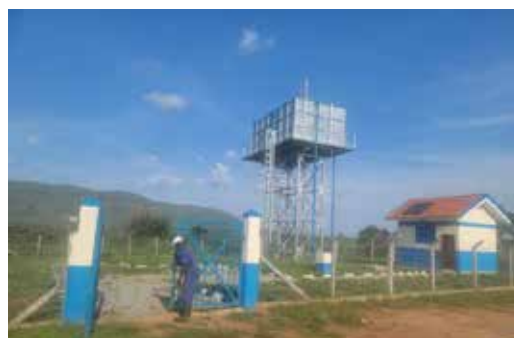
Reservoir tank, chlorine dosing house for Arra/Dufille WSS in Moyo District
