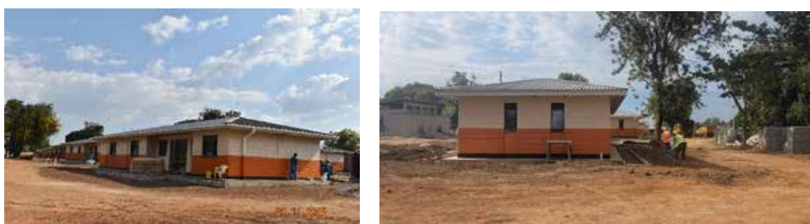
Staff quarters under construction as part of additional works at Busolwe General Hospital
