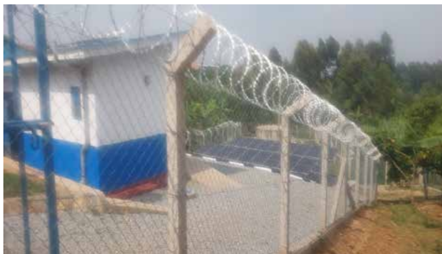
Water supply scheme upgraded with a solar system in Masheruka, Sheema
