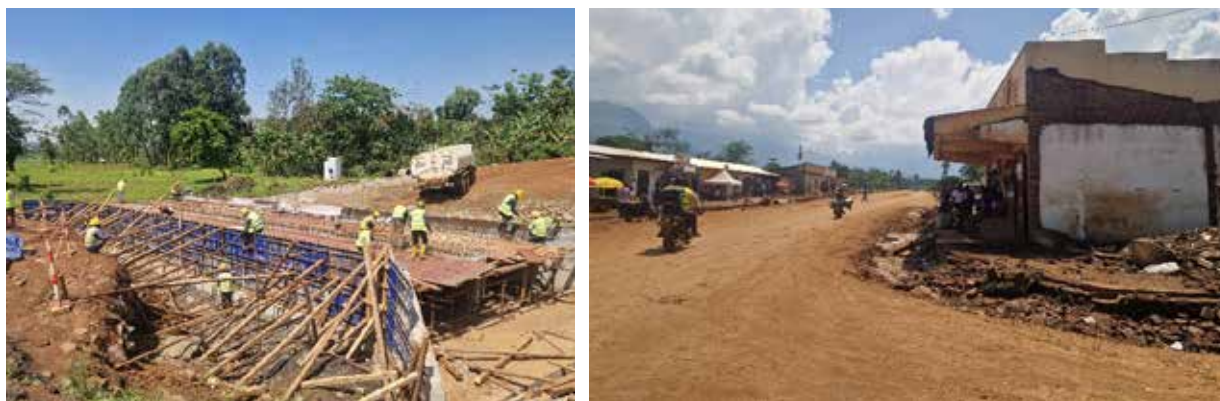
Namagumba – Budadiri – Nalugugu Road, L-R: Construction of a two-cell box culvert at km 8+4580; Structures in the construction site due to compensation issues
