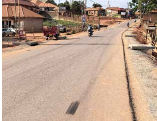
A section of Lubugumu-Kakola road with asphalt pending the construction of walkways in Makindye Ssabagabo Municipality
