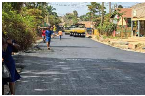
Ongoing construction of the asphalt layer on Kisaasi 2 road under Lot 4 in Nakawa Division
