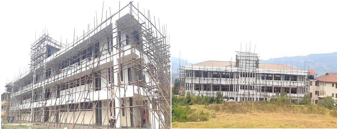
A front and rear view of the 3-storeyed Science Lecture Block under construction at Kabale University at 82% progress
