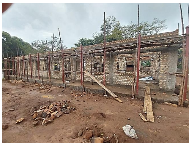
Ongoing construction of the multi-purpose hall at Kitagobwa UMEA Primary School in Butambala District
