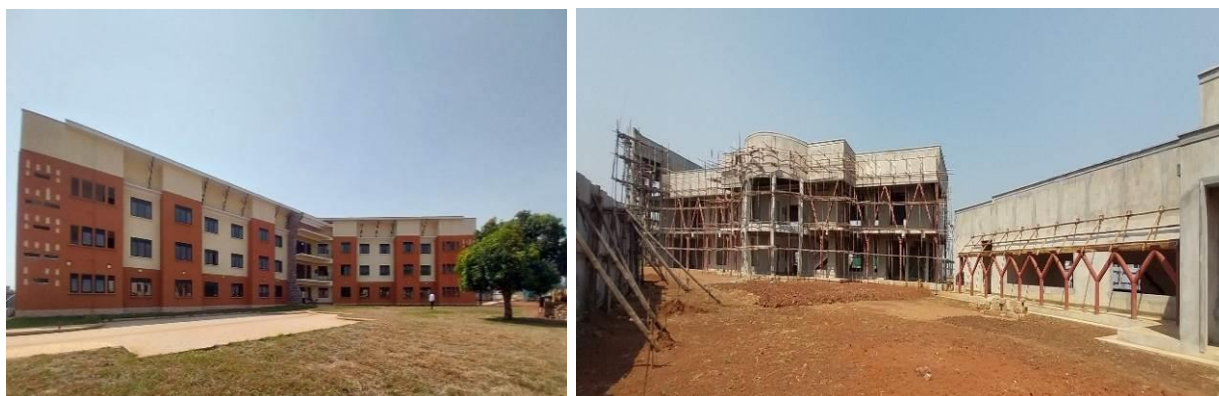
Left-Right: Stalled female hostel block, and the lecture block at Uganda Petroleum Institute Kigumba in Kiryandongo District at 80%
