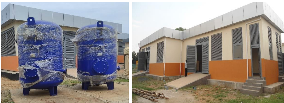
L-R: Uninstalled equipment at Soroti RRH and Plant House at Hoima RRH
