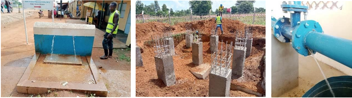
L-R: A PSP of Atiak WSS in Atiak Town Council in Amuru District; Stud columns for the reservoir tank; and a leaking flange of Bulangira WSS in Kibuku District
