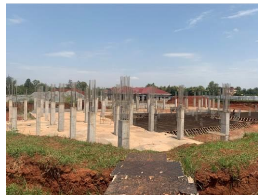
The six-floor Business Development Centre/Centre Teaching Facility stalled at 20% progress at Gulu University
