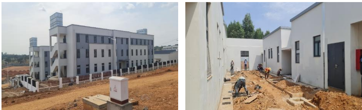
L-R: Substantially completed boy's hostels. Incomplete external works at the staff quarters at the NSTEIC at Rwebitete-Kiruhura District
