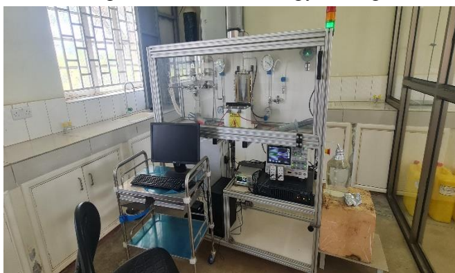
On site air-to-fertilizer mini-plant prototype installed in a laboratory at Kamenyamigo Satellite Station-MUZARDI in Lwengo District
