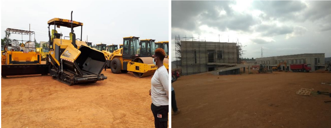
L-R: Some of the construction equipment for the TSC and progress on civil works at NSTEIC-Rwebitete
