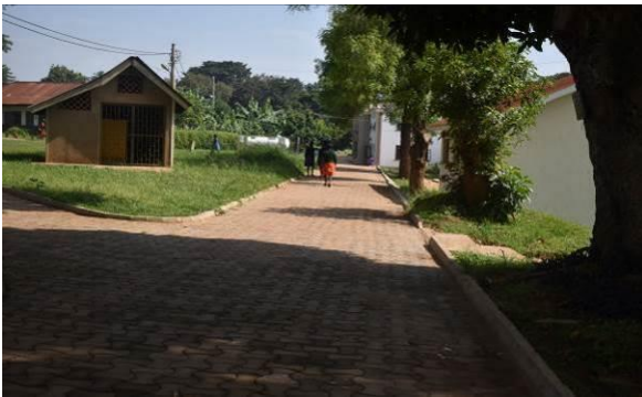
One of the completed walkways with pavers and kerb lines at Gayaza High School in Kasangati Town Council
