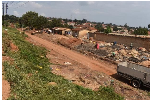
A compacted section where the old rail tracks were removed at Namboole
