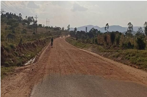
Mbarara UNRA Station: A well-graded and shaped section at the start of the Kikagati-Kafunjo (30kms) Road
