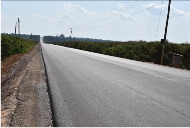
Mityana-Mubende Road: Asphalt surfacing between Kms 11 to 12 with a site toilet in the background
