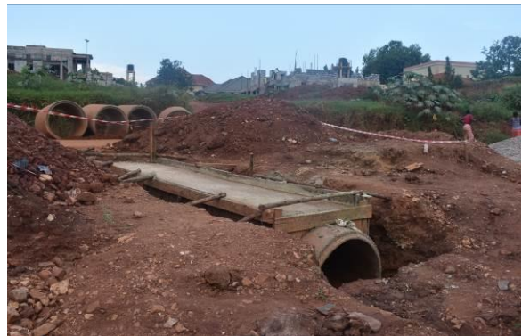
Installation at half road with an encased concrete pipe culvert installation of 900mm diameter along the Shimoni PTC (3.4kms) Access in Kira Municipality
