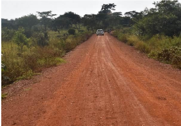
DRRU-Central: A completed section at Kms8+000 on Bbaale-Gira-Kanyogoga (10.3kms) used as access to the Bulwandi-Gyra swamp crossing from the Kayunga side.
