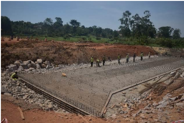
Foundation works for a box culvert along the Kasangati –Matugga Section on the Kira-Matugga Road Project
