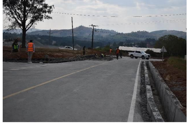
Ongoing works on one of the Kyamate Access roads in Ntungamo Municipality
