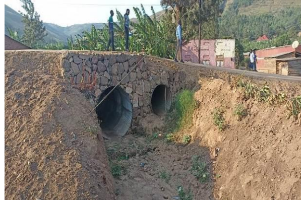
Mbarara UNRA Station: 1.8m and 1.2m Armco culverts installed with gabion end structures at Ruborogota TC along Kikagati-Kafunjo (30kms) Road At Kms 10
