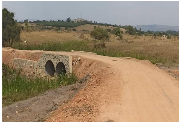
DRRU-West: A well-raised swamp section with two 1200mm diameter Armco culverts with headwalls along Mile 8-Katojo-Rwentanga T/C (5.2kms) Road in Mbarara District
