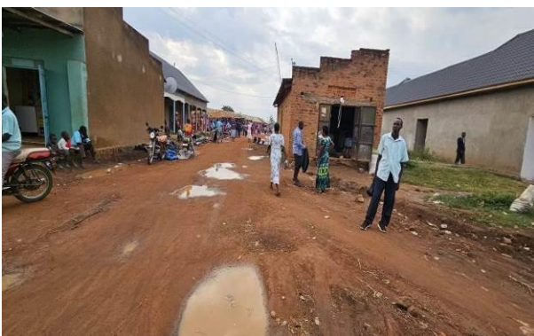
Unstabilised base and house on RHS within the road alignment at Kibuku TC roads along Market Street Road
