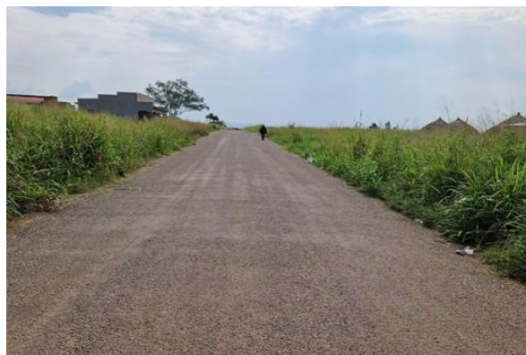
Amuru District: Market Street in Pabbo TC was upgraded using low-cost seal technology
