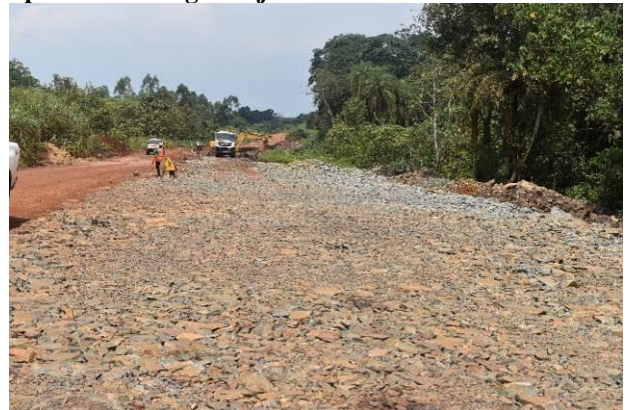
Rock fill in a section with a high water table in the Budongo Forest at Kms 31+620 along the Masindi-Biiso (43kms) Road Project on Oil Road Package 5
