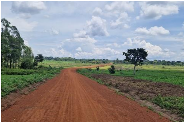
DRRU-Jinja: Bubinga-Buyebe-Buwabe Road (6.5kms) in Bugweri District after the rehabilitation works. The swamp section was raised.
