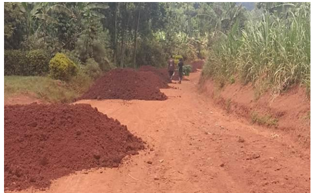
Lugazi Municipality: Gravel heaps damped on a graded and shaped section of Dangale-Kimwanyi road in Najjembe Division
