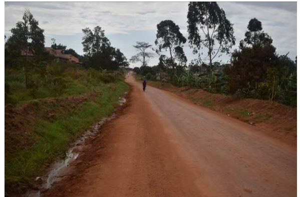
Mpigi UNRA Station: A well-formed shaped section with a surface in good condition of Mitalamaria-Bulo-Kanoni Road at kms 27+800
