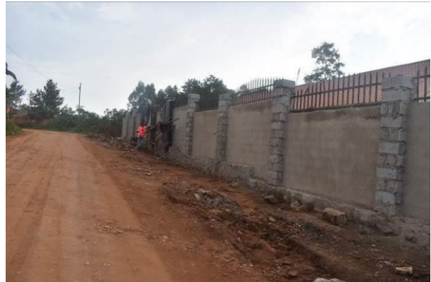
Ongoing construction of a boundary wall aimed at widening the road at Kms 2+680 along the Bulindo-Nsasa-Namugongo (4.56kms) Road in Kira Municipality
