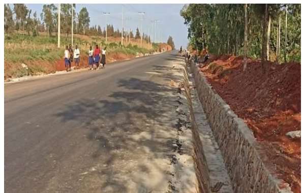
Ongoing stone pitching works of the side drains in a section that has received asphalt at Kms 2+580 long Kafunta-Buwampa Road (9.5kms) in Njeru Town Council
