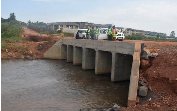
A 2.5m by 2m six-cell box culvert in a swamp crossing along the Kitukutwe-Kiwologoma (4.54kms) road in Kira Municipality
