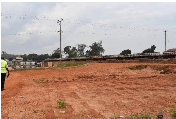
Assembled rail tracks loaded on a train at Kawolo-Lugazi for transportation to Kampala-Namanve section works
