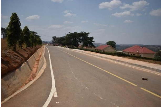
One of the completed Rushere Town roads with a pedestrian walkway, concrete line drain, and road markings
