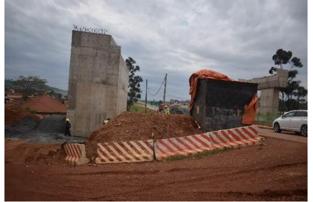
The abutment and pier works for the Lweza-Lutembe Vehicle Overbridge at Kajjansi along the Munyonyo Spur on the Najjankumbi-Busabala and Munyonyo Spur Interchange Project
