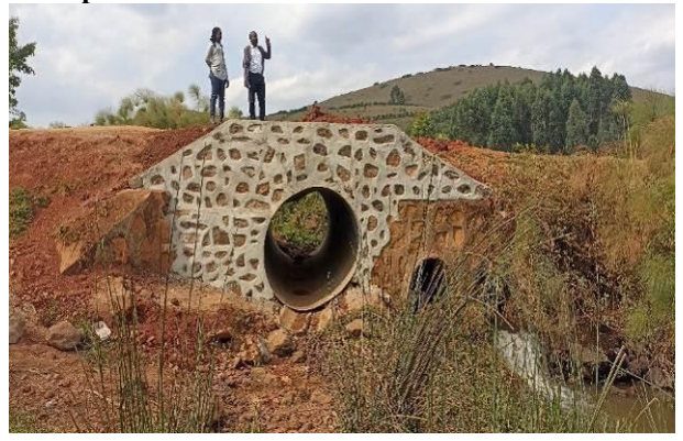
Ntungamo District: The 1800mm diameter Armeo culvert along the Katinda-Kagrama Road at kms 1+000
