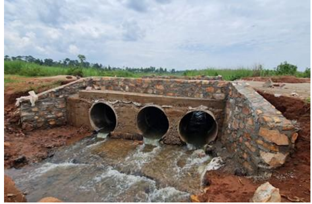
Jinja District: Three lines of concrete culverts installed on Busoona- Budiima road at Nabukosi swamp
