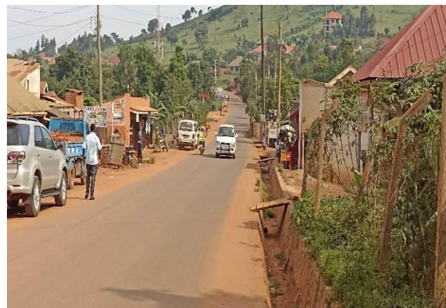
A completed paved section with a stone-pitched side drain on the Nansana-Kireka-Bbira Road in Nansana MC constructed using Probase Technology
