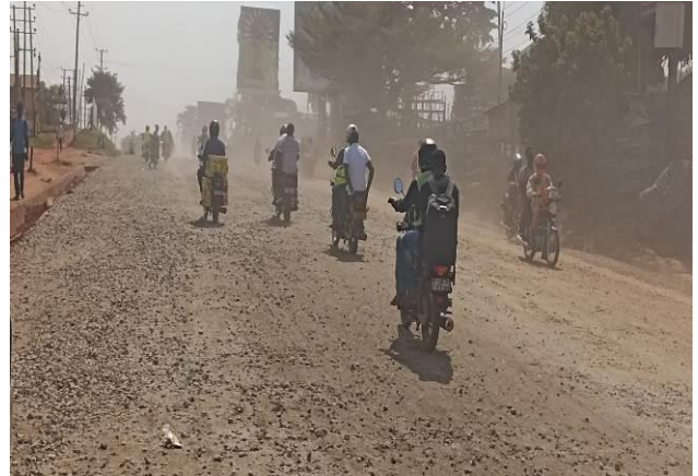
Kampala-Jinja Road: CRR works at the start of the project at Nakawa
