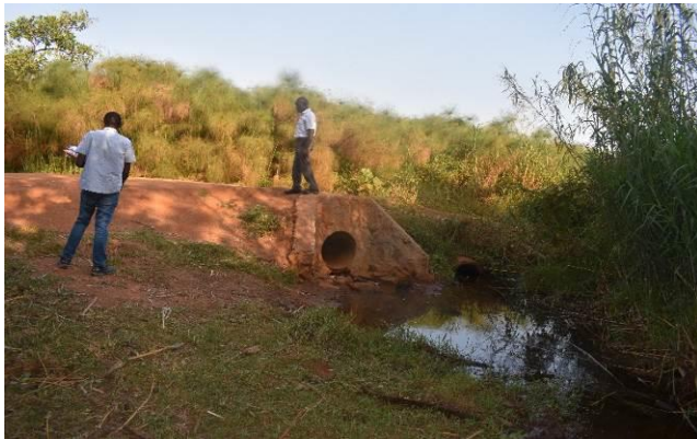
Kakumiro district: A culvert installed at a section along Bukuumi-Kibijjo-Isunga Road at kms 2+000
