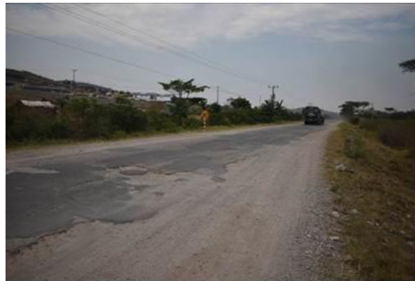
Kasese UNRA Station: A section of Kikorongo-Mpondwe road that was patched with gravel at kms 6+000
