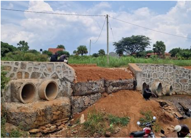
Gulu UNRA Station: Culverts installed along Gulu – Airfield road (4kms) as part of emergency intervention
