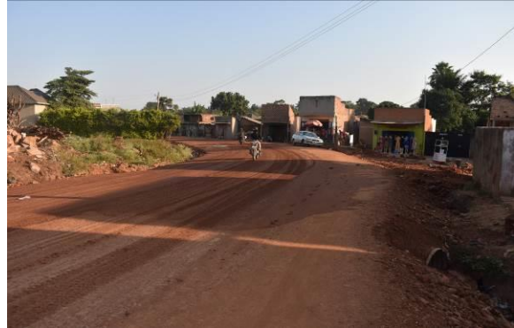
A prepared subbase layer in preparation for surface dressing and an installed Armco culvert without end structures along Matu Road in Busunju Town Council
