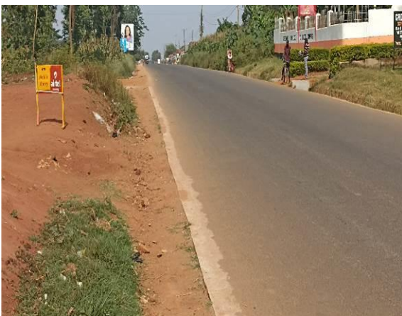
A completed paved section with a concrete edge beam in Kayunga Town on the Kayunga-Nabuganyi Road in Kayunga District using the Probase Technology
