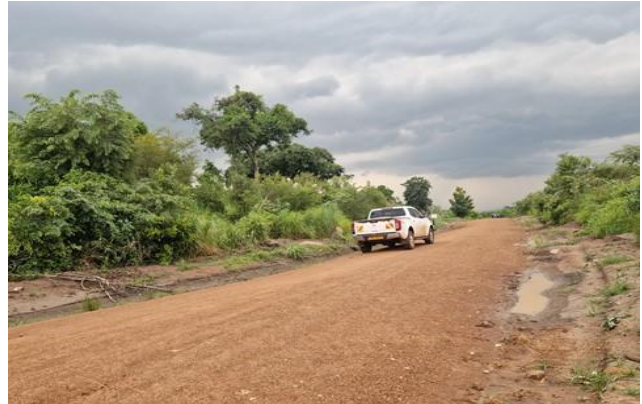
DRRU-North: Ibibiaworo Pakele road (7kms) was rehabilitated in Adjumani District (fully gravelled)
