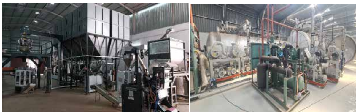
Some of the equipment installed at Inspire Africa Coffee factory at Rwashamire-Ntungamo district.
