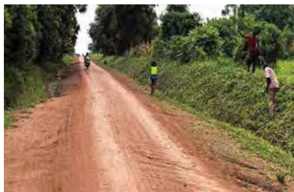
Lira MoWT Station: A graded section at km 10+100 with a deteriorated surface along Lira–Boroboro–Aboke (41 km) under framework contract
