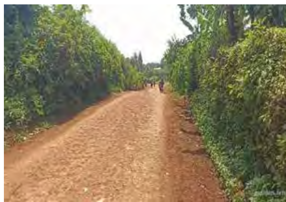
Kween District: A deteriorated graded section at km 2+000 along Atari-Mokotyo Road (14.5 km) using the Road Maintenance Grant
