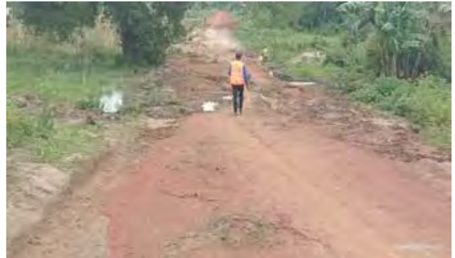
DRRU-North: A low-lying section yet to be worked on at km 2+800 long the Alooi–Ogini–Kakira PS Road (3 km) in Alebtong District
