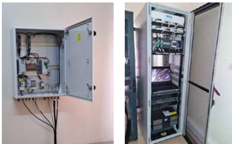
Server cabin (left) and wind shear cabin (right) at the National Meteorological Centre in Entebbe
