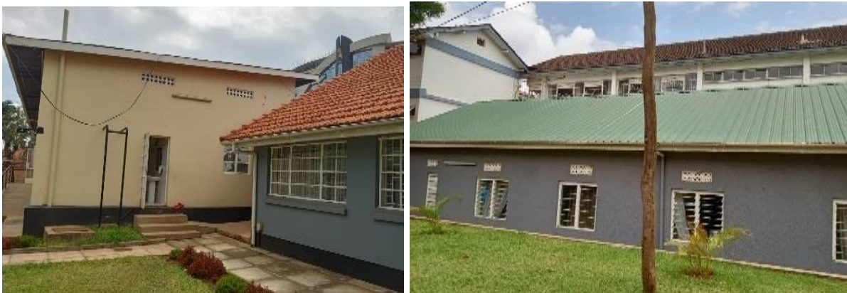
L-R: Renovated Pension Registry and Accounts Block; Renovated green roof at the Ministry of Public Service Headquarters
