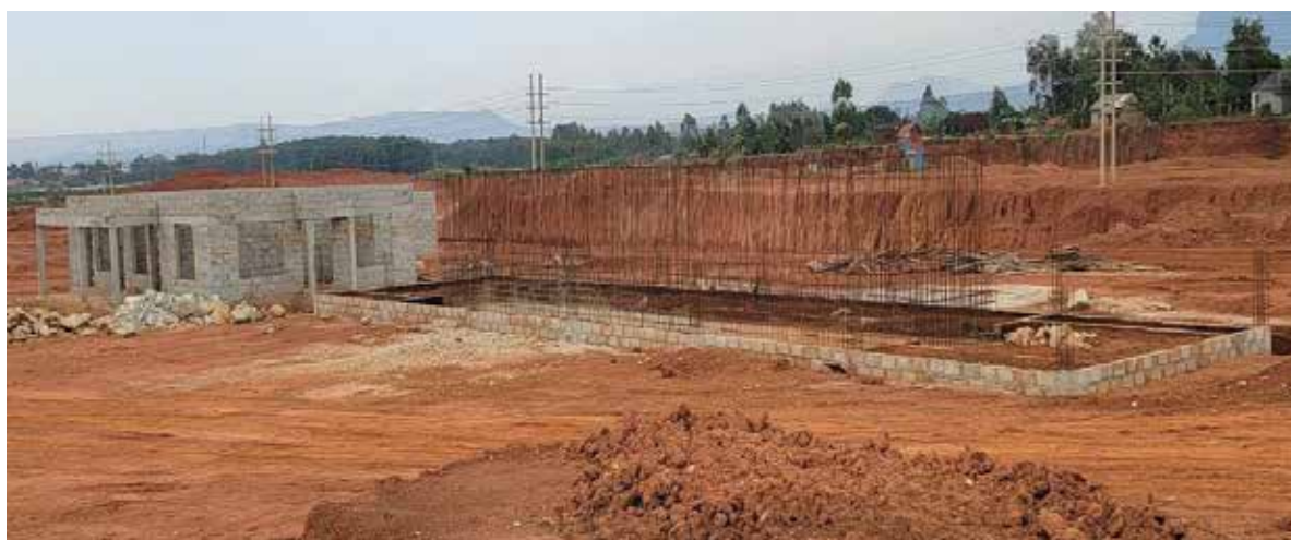
Stalled works at the waste water treatment site in Sino-Mbale industrial park, Mbale City
