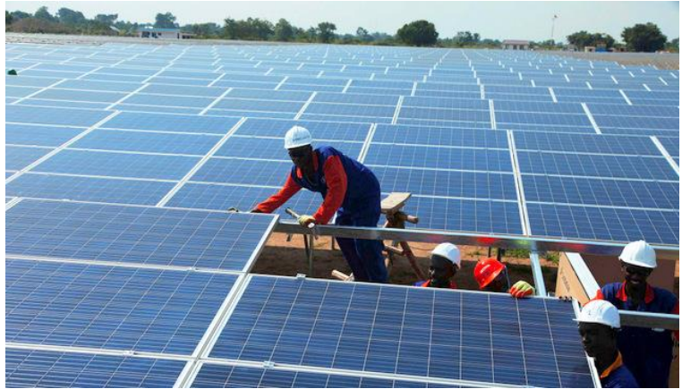
Technicians undertaking final installation works on panels for the solar generation plant at Busitema, Busia District
