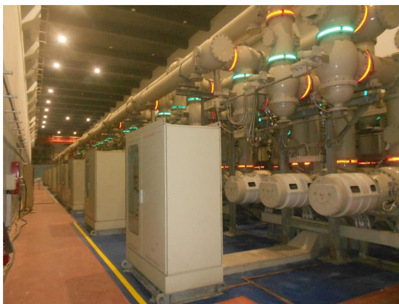
Newly re-installed electrical cubicles in the Karuma HPP Powerhouse
