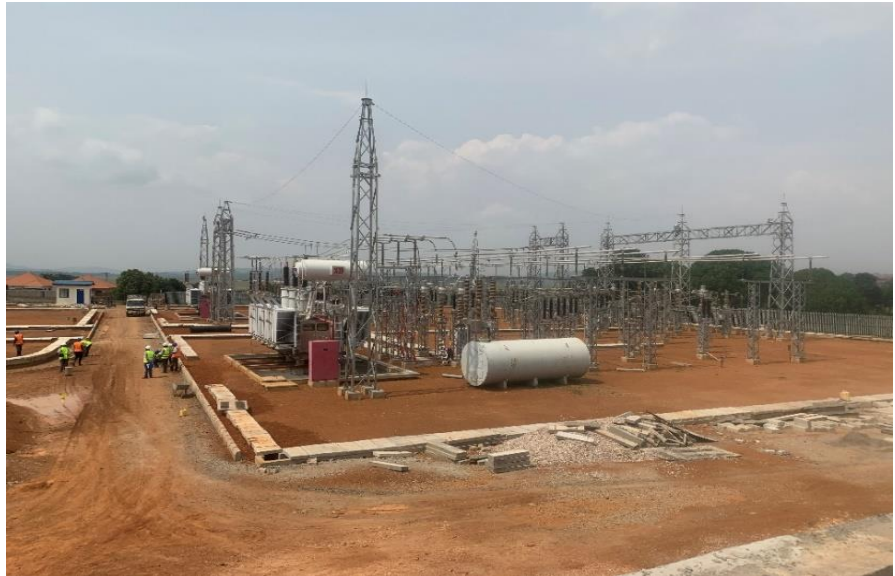
Partially completed Entebbe Substation Switchyard
