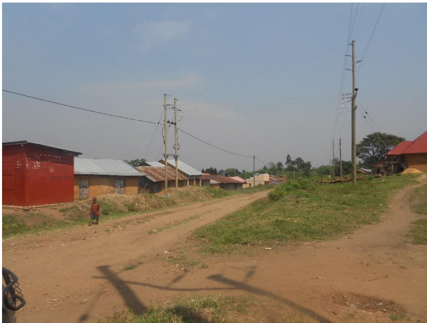
Ongoing grid extension scheme under ERT III in Omukitunzi TC, Kanungu District
