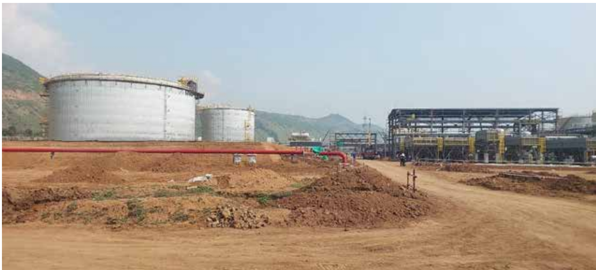
Completed crude oil storage tanks at Kingfisher CPF in Kikuube
