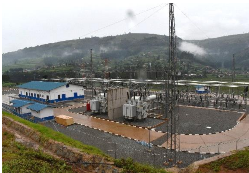
Completed Kabale 132 kV substation
