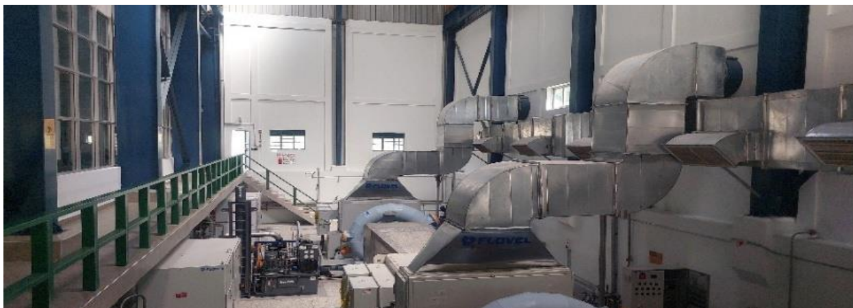
Installed electromechanical equipment in the Nyagak III Power house
