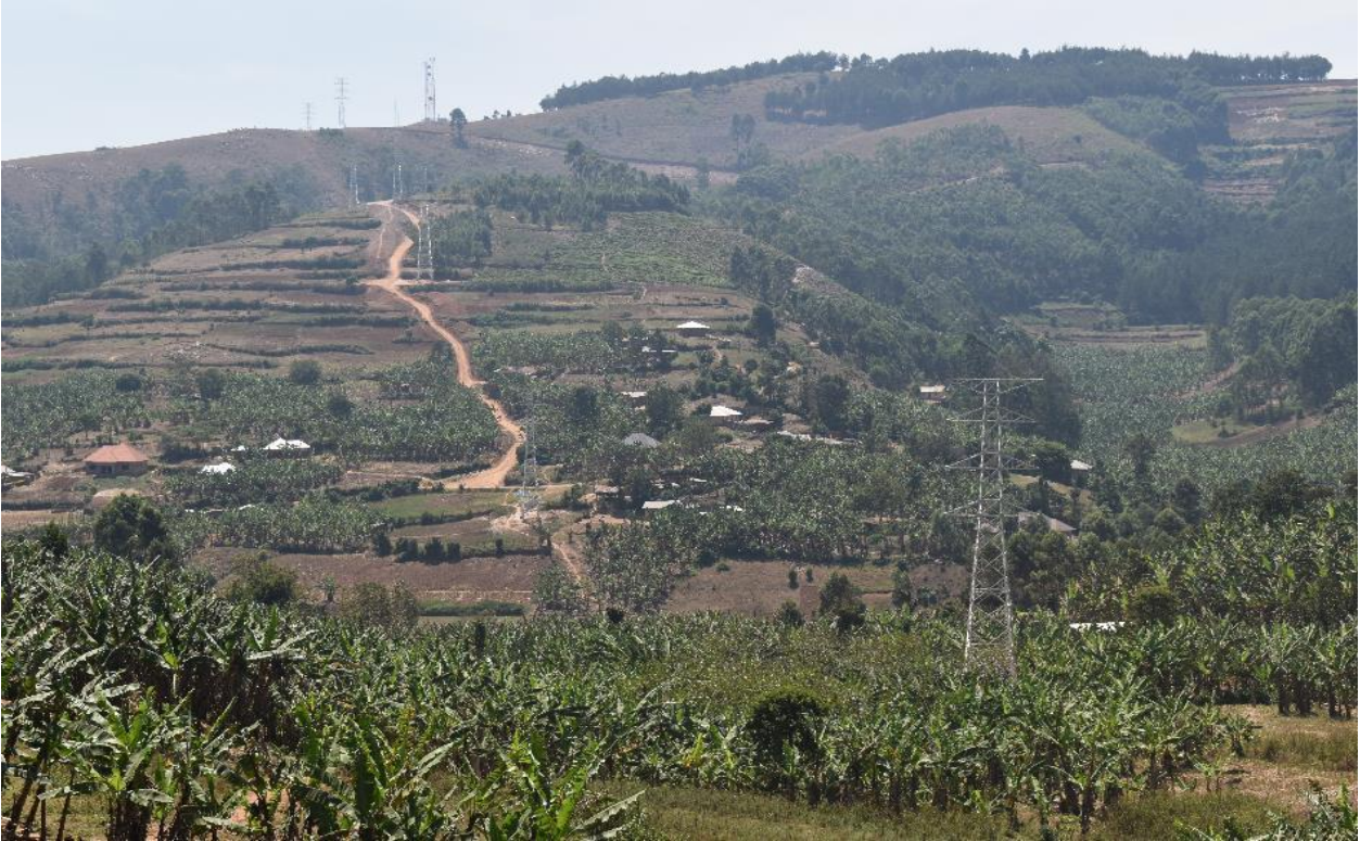
Completed towers on a section of the Mirama-Kabale Transmission Line in Kabale District
