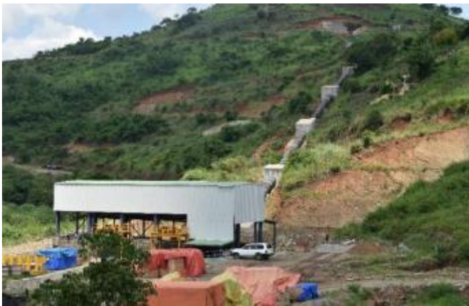
L: Completed penstock and partially completed plant house building at Nyagak III HPP
