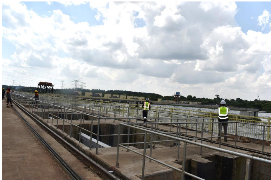
R: Karuma HPP intake section, with missing log boom
