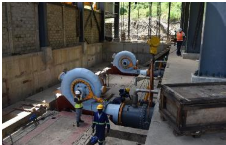
R: Ongoing electromechanical installation works on the turbines at Nyagak III HPP powerhouse
